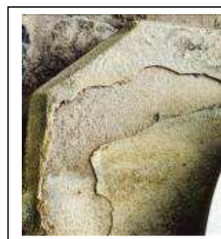
Figure 80 Minor scaling and flaking
