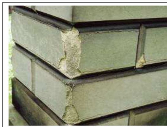
Figure 77 Moderate contour scaling on flat surface
