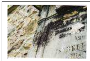
Figure 82 Major pollution staining
