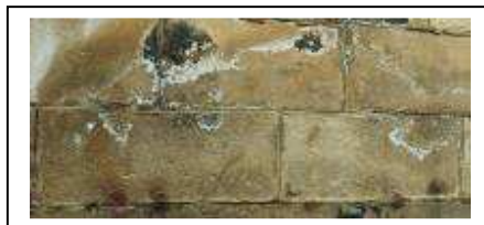
Figure 81 Major salts deposit
